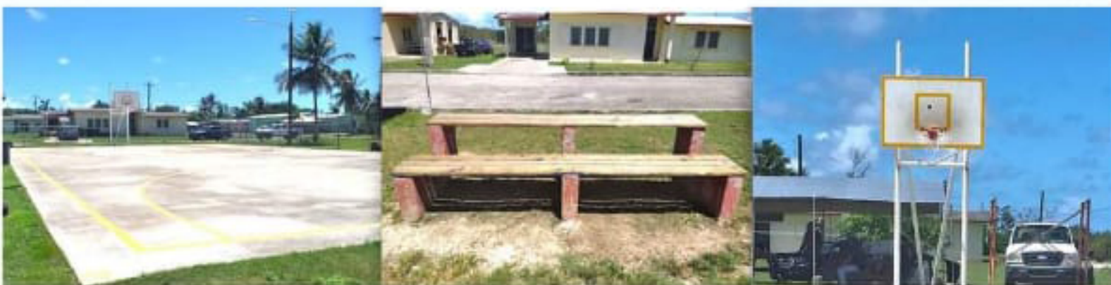
CONTRIBUTED PHOTO This combo photos shows the Broadway Estates Basketball Court and its features before undergoing transformation.
